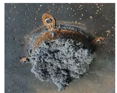
Seal impermeable to fire and hot gas after the fire protection collar is activated.
