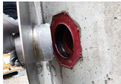
3. Apply lubricant to the spigot end and slide it in as far as it can go.
